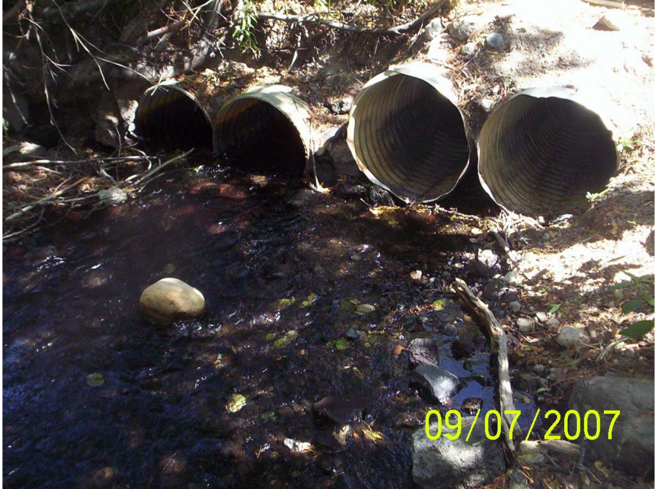
Figure B-4. A culvert installed in Reach B of Mammoth Creek as part of a driveway to provide access to a private residence.
