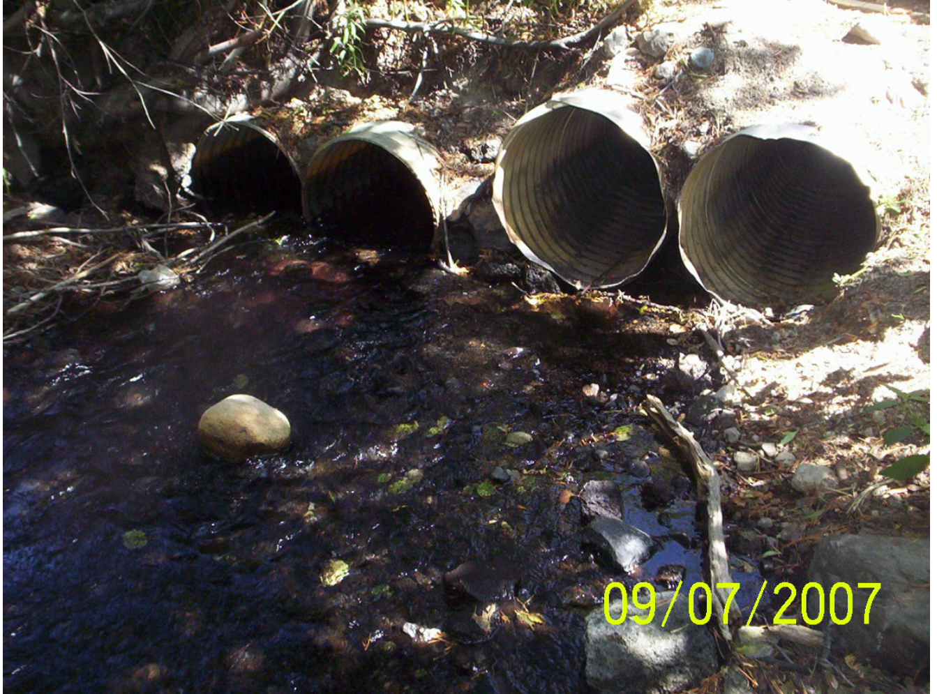
Figure B-4. A culvert installed in Reach B of Mammoth Creek as part of a driveway to provide access to a private residence.
