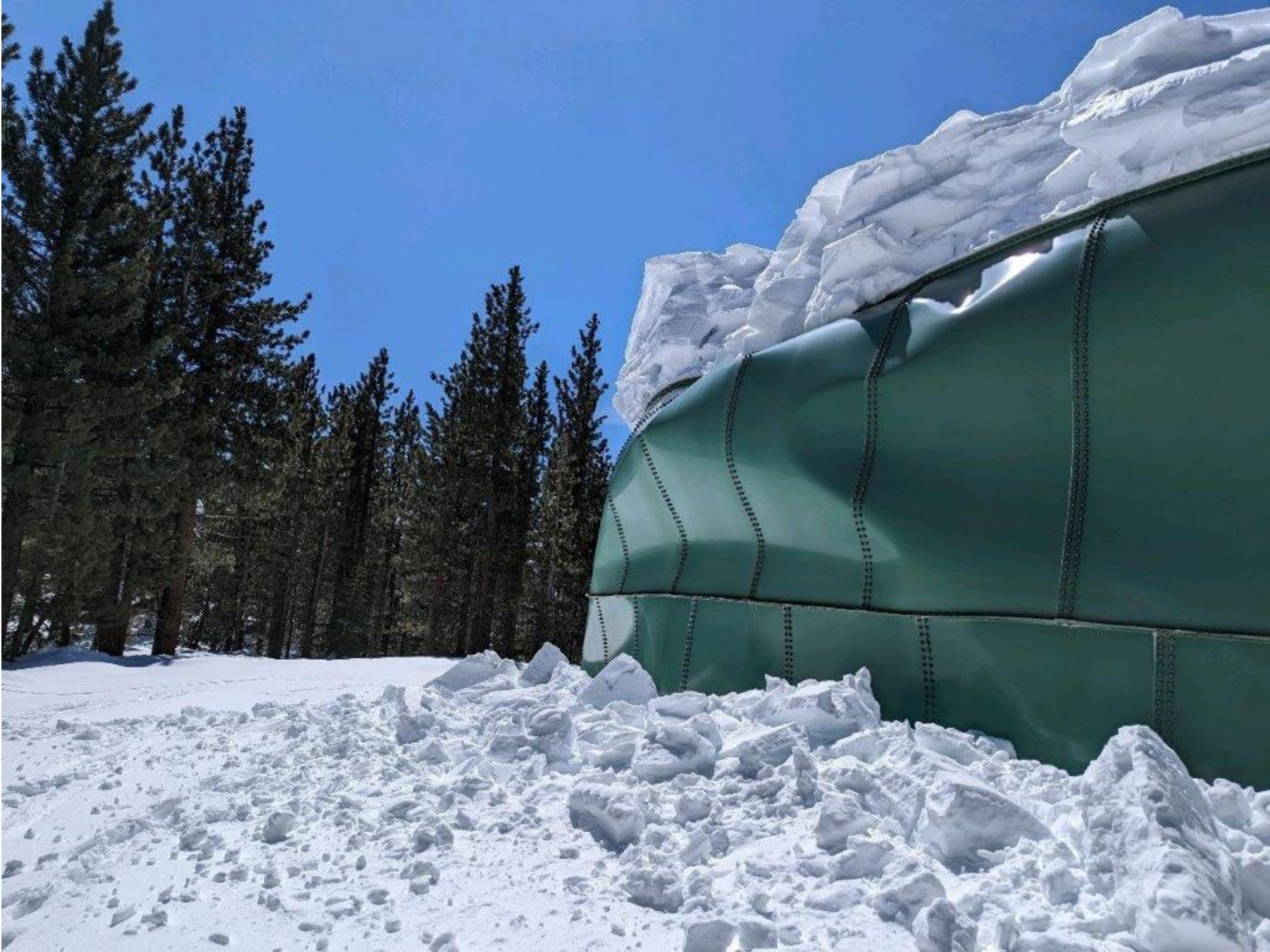
Tank T8 (Forest Trail) Failure, 2023
