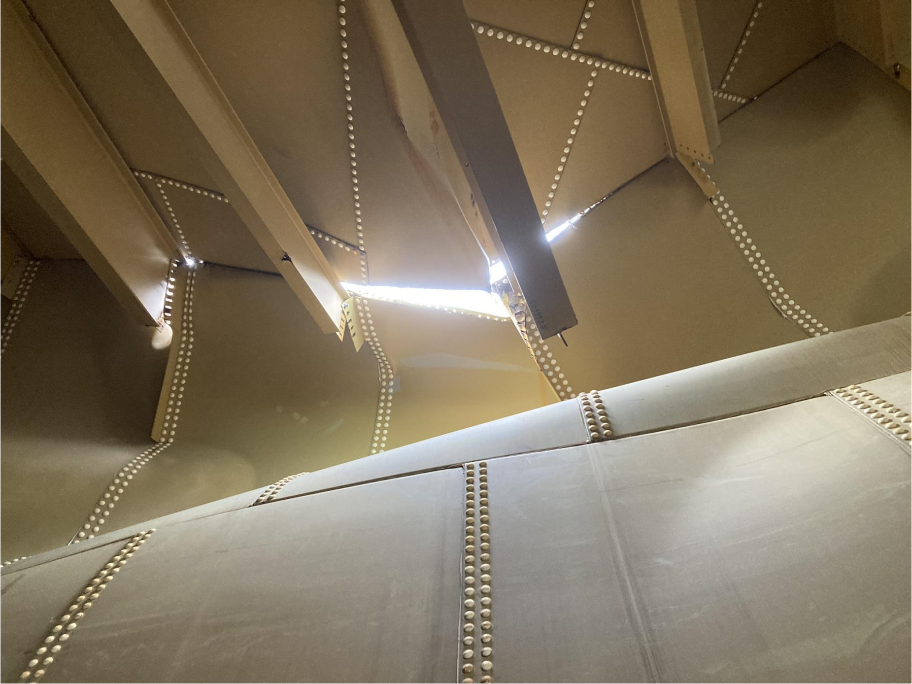
Tank T8 (Forest Trail) Failure, 2023
