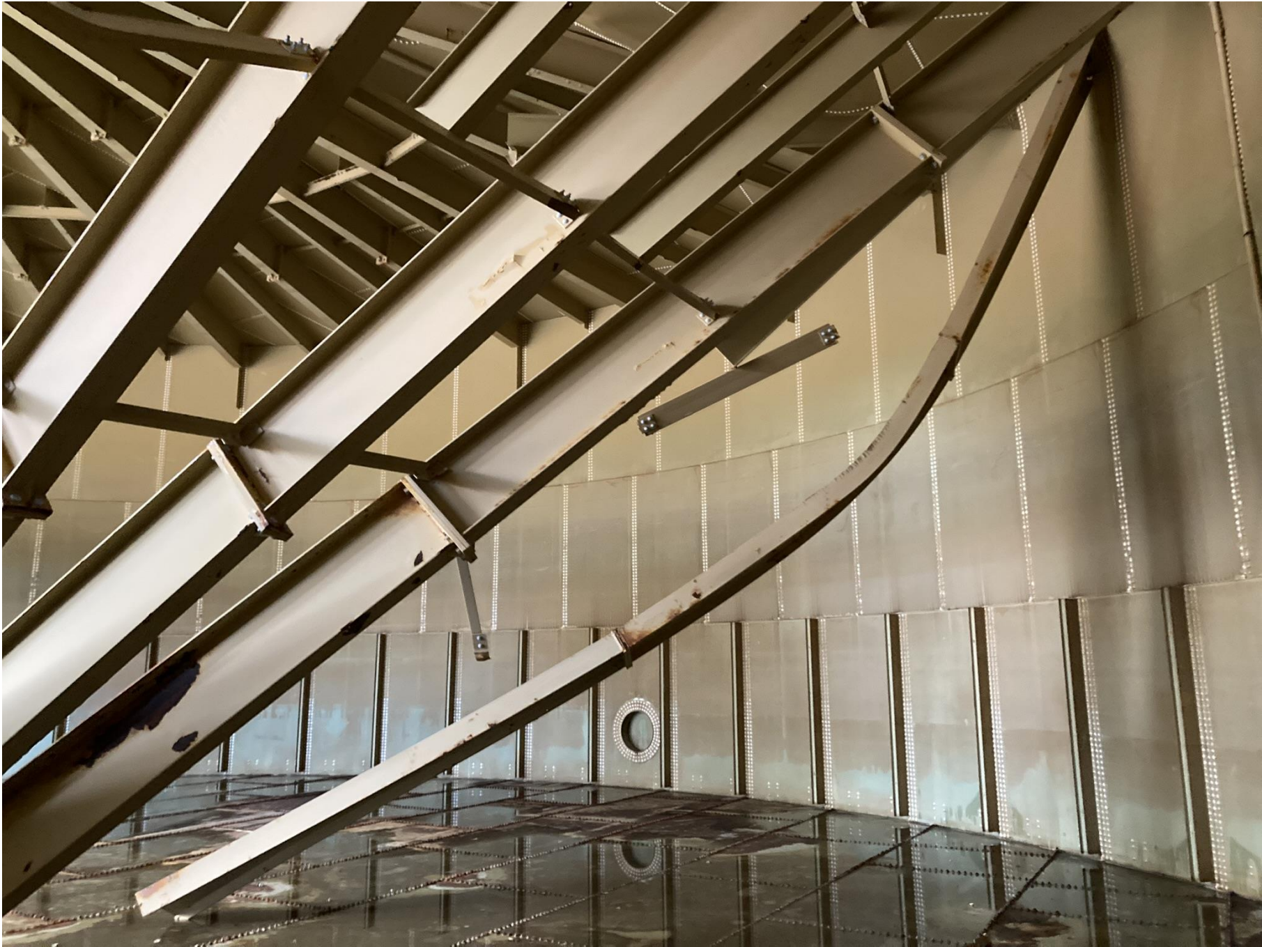
Tank T8 (Forest Trail) Failure, 2023
