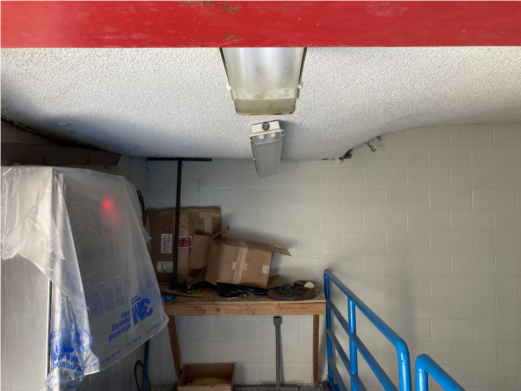
Equalization Pumps Building Partial Roof Collapse, 2023
