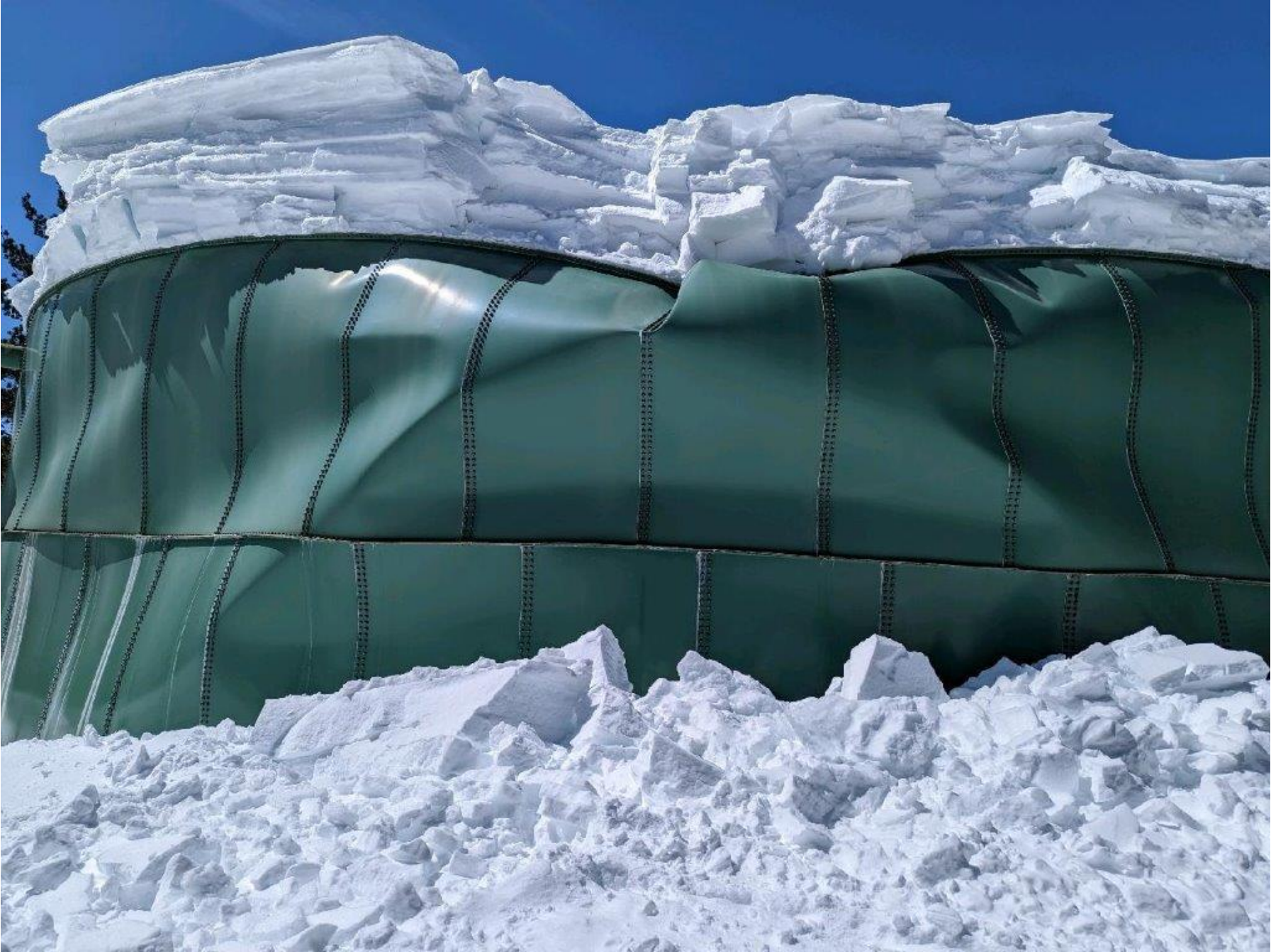
Tank T8 (Forest Trail) Failure, 2023
