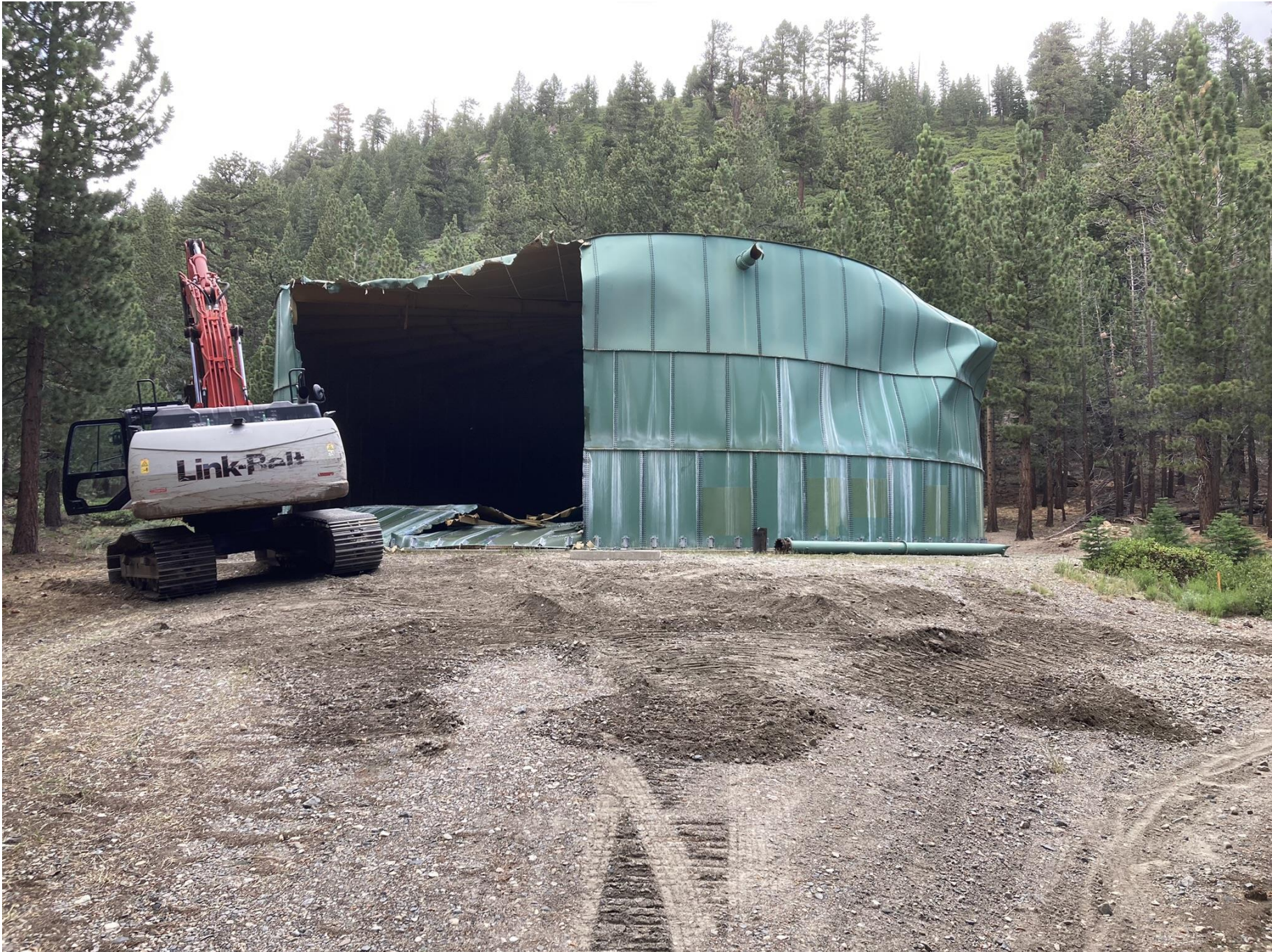
Tank T8 (Forest Trail) Failure, 2023
