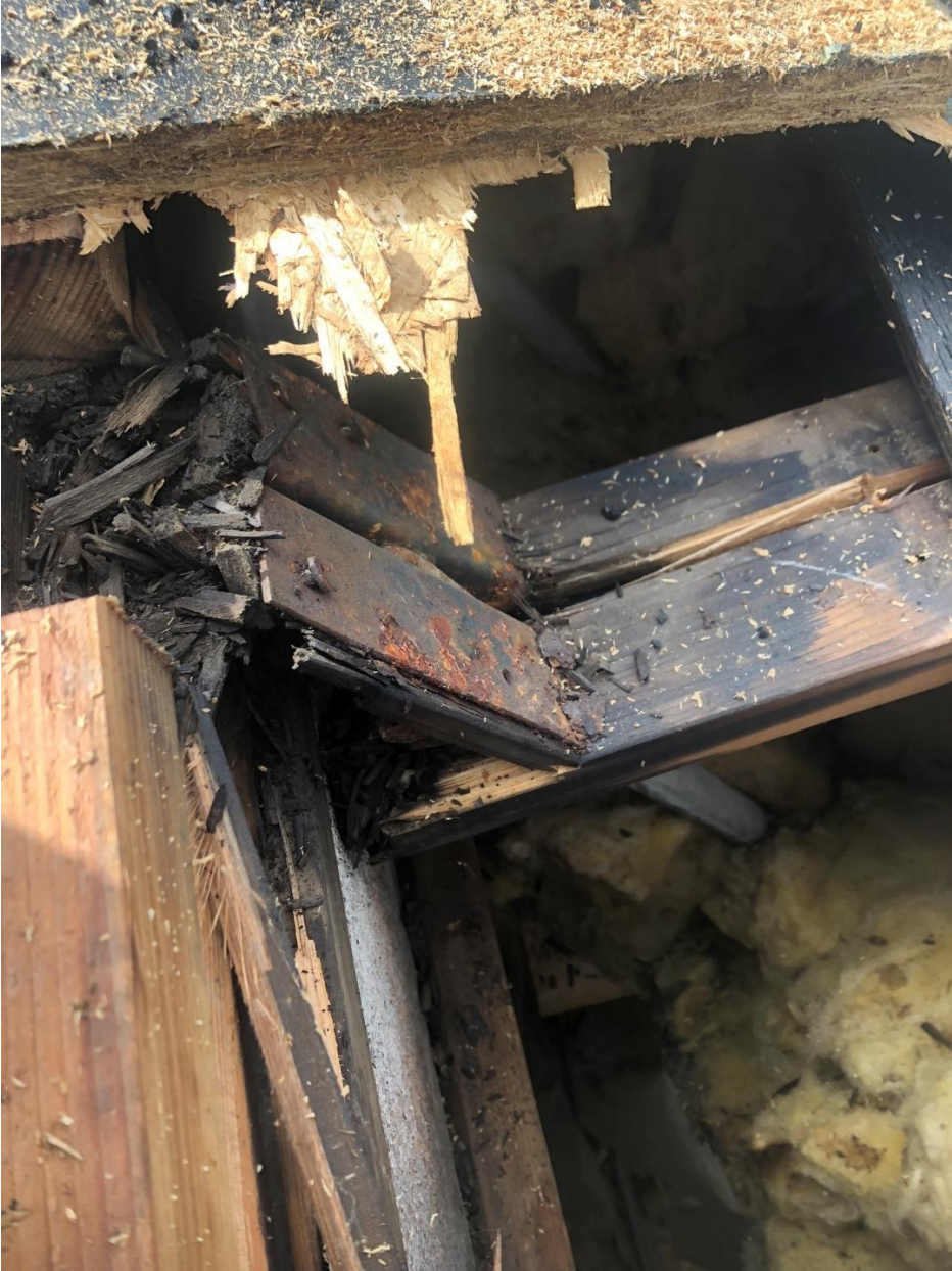
Equalization Pumps Building Partial Roof Collapse, 2023
