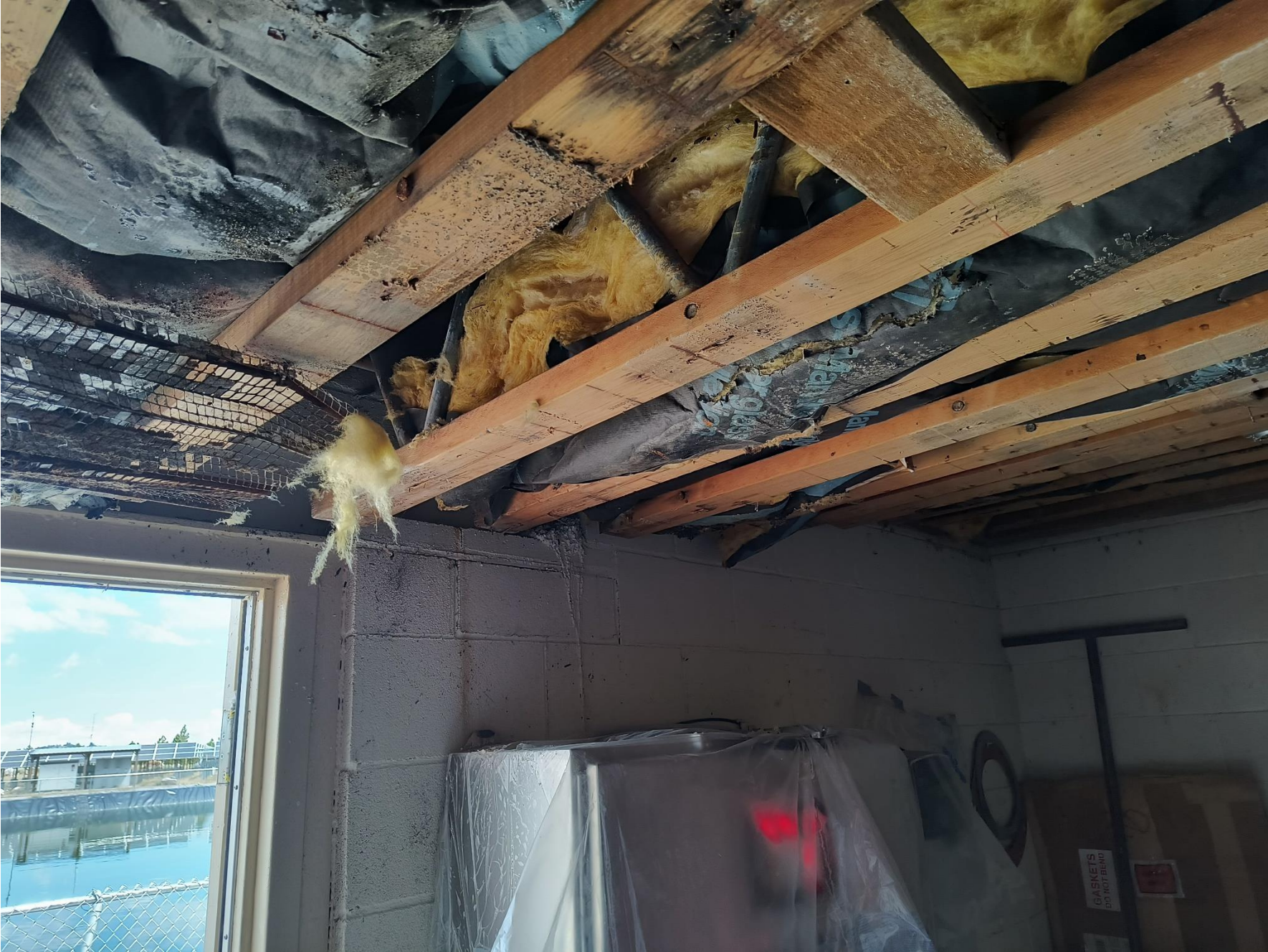
Equalization Pumps Building Partial Roof Collapse, 2023
