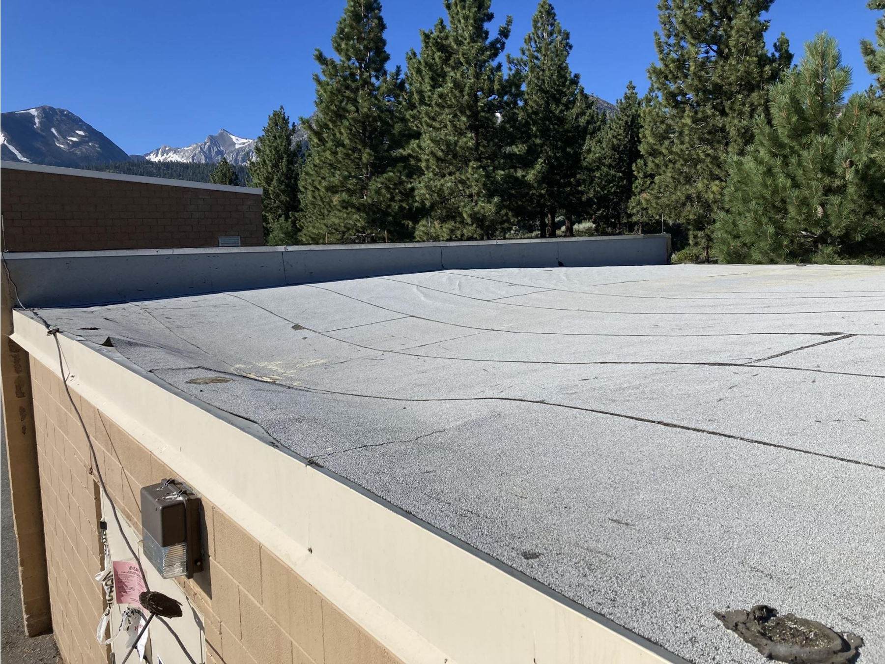
Equalization Pumps Building Partial Roof Collapse, 2023
