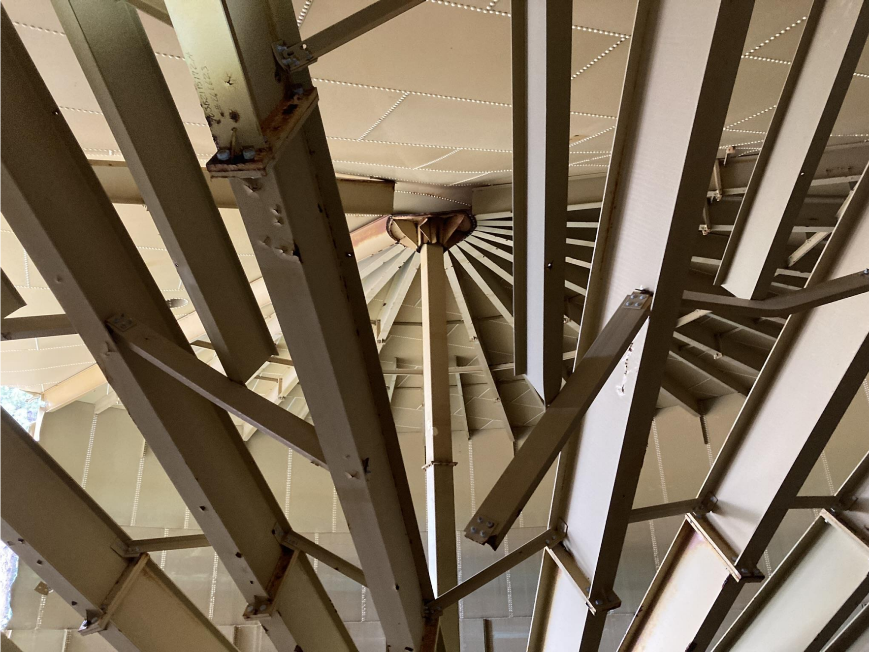
Tank T8 (Forest Trail) Failure, 2023
