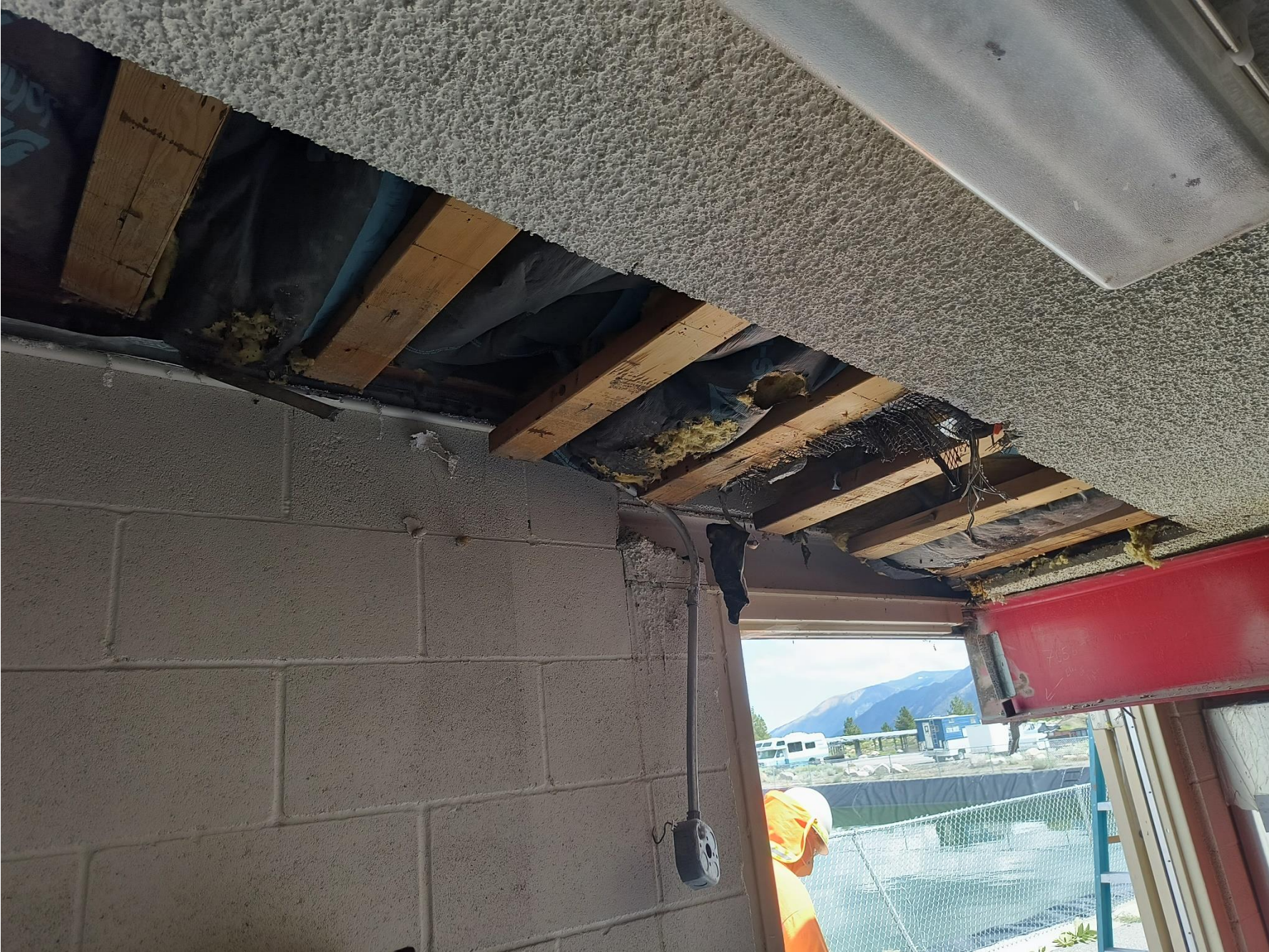
Equalization Pumps Building Partial Roof Collapse, 2023
