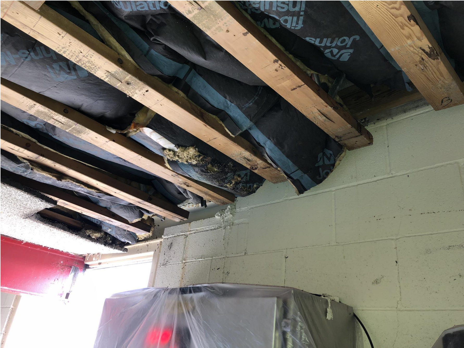
Equalization Pumps Building Partial Roof Collapse, 2023
