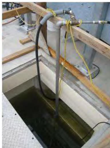
Figure 4: Effluent Sampling Location at LAWRP
