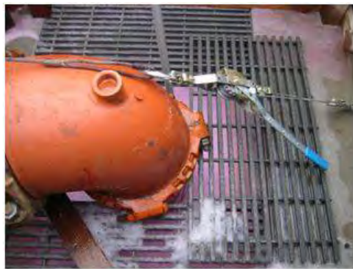
Figure 3: Tracer Injection Location (CCT Influent Box) at LAWRP
